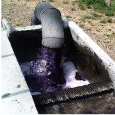
....chemicals in the effluent
